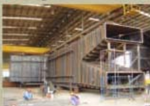
▼ Rabigh - Boiler Duct
