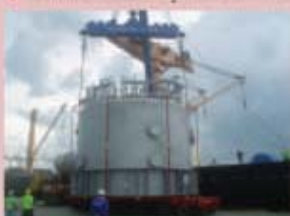
▼ Shadeed DRI - Top Gas Scrubber
