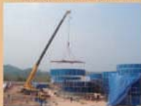
▼ Sepon Copper-Duplex Tanks
