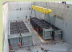
▼ Connectiv, PA, USA
