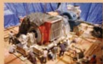
▼ TPI Ethylene - Steam Turbine
