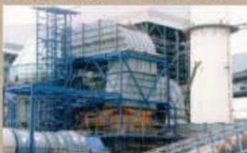
▼ Maemoh 4 - 7 - FGD Ducts
