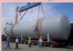
▼ Shadeed DRI - Purge Gas Tank
